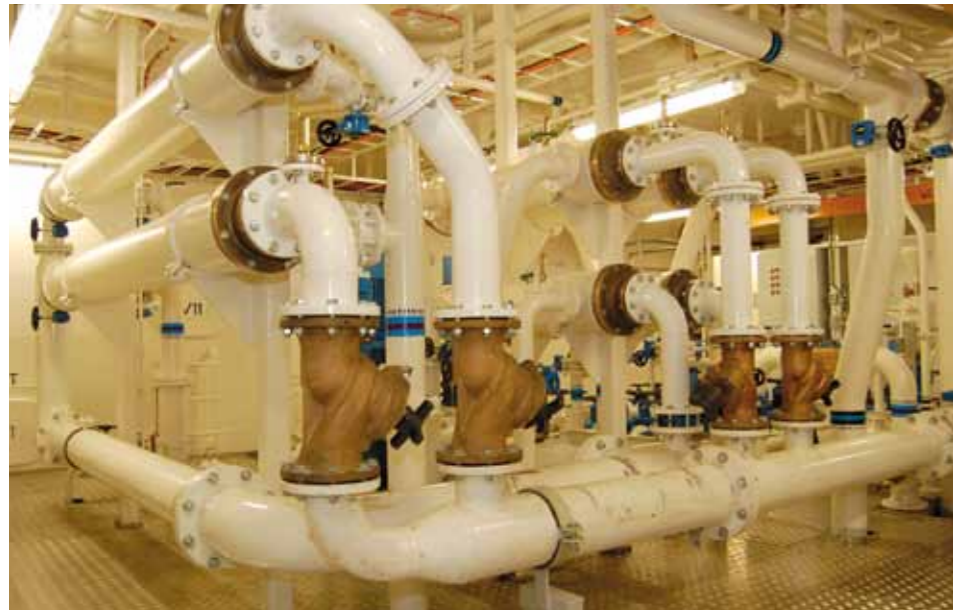
The pump room is a work of art for engineers
