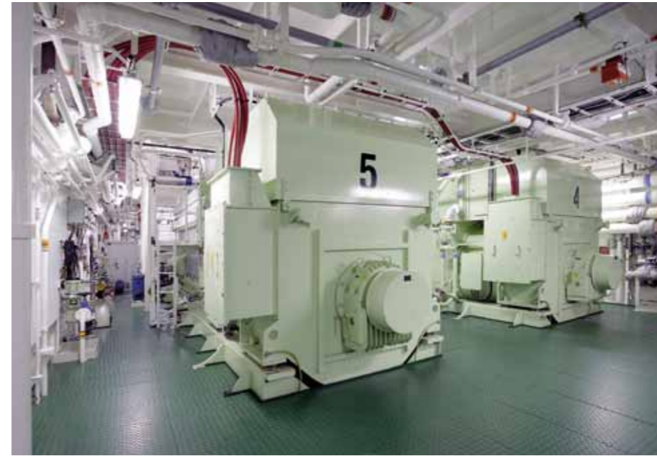
The electrical installation comprises of an energy system with 6 board net transformers, feeding a low and high voltage installation
