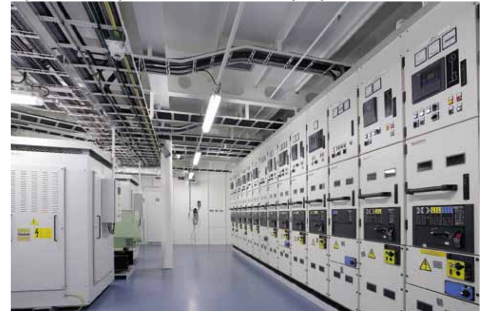
The power is distributed through two main switchboard rooms with low and high voltage circuits
