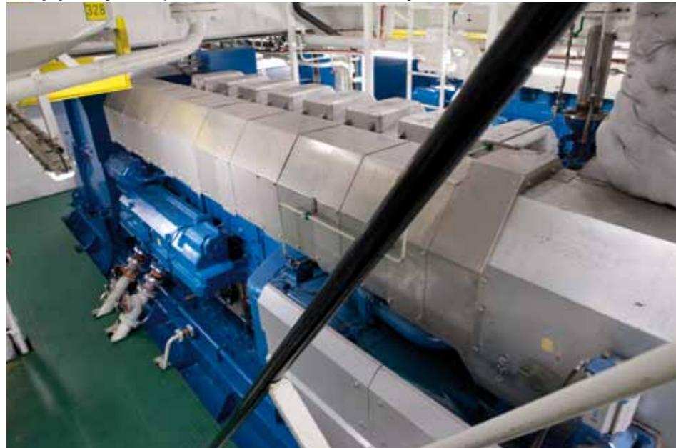
The ship's power is generated by two times three 3,840 kW (4,100 kVA) diesel generator sets
