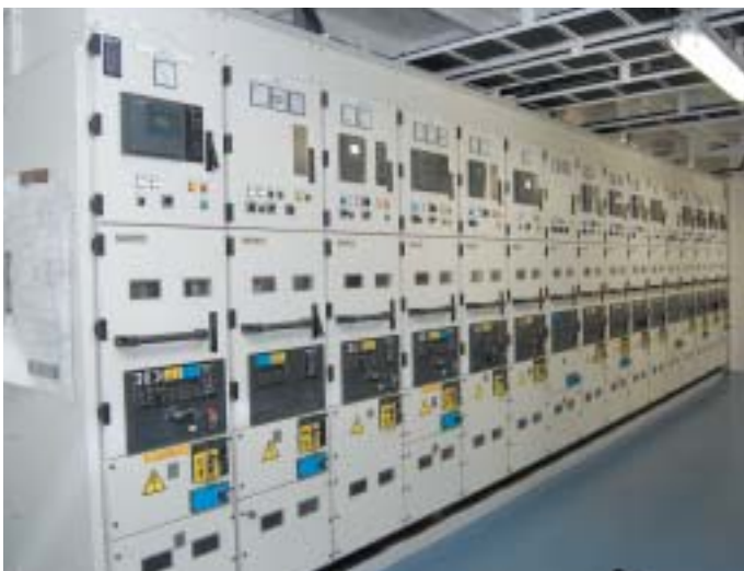
The main switchboard is the heart of the diesel-electric propulsion installation
