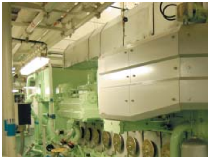
Six Wärtsilä dual fuel engines provide a total of 20.160 kW
