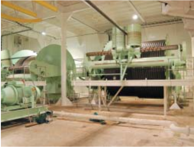
The A & R winch is located below the aft deck
