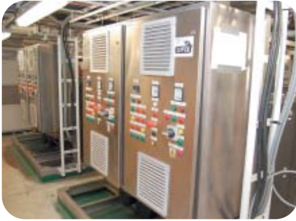
The diving control system uses remote operated valves
