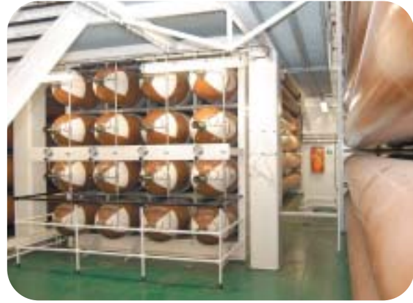
A large supply of helium/oxygen mixture is stored under deck
