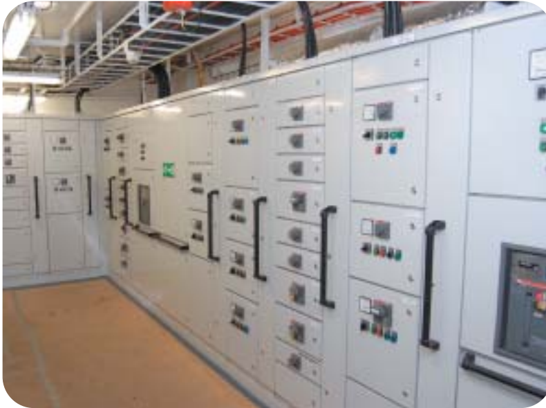
All propulsion equipment is fully redundant to achieve DP-3 class
